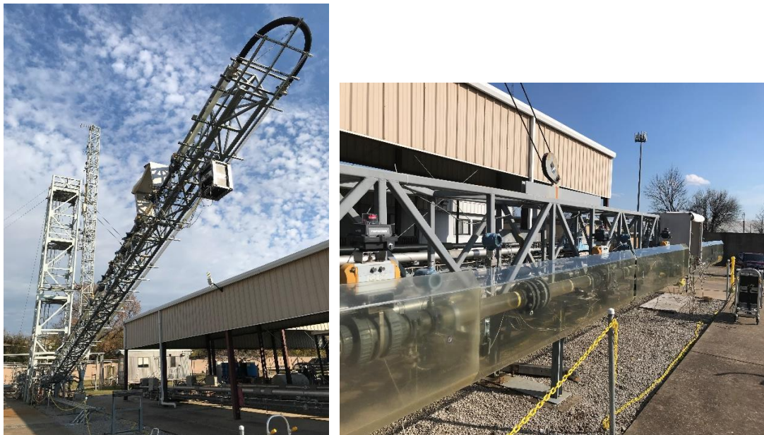
Figure 4: Pictures of the 4-in facility.
